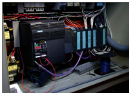
A SIEMENS MICROMASTER AC DRIVE CONTROLS A 1 HP MOTOR/PUMP COMBINATION FOR FLOW AND APPROPRIATE SPEEDS FOR THE BAKING MOTION INSIDE THE LAUTER TUN AFTER IT HAS RECEIVED THE MASH.
